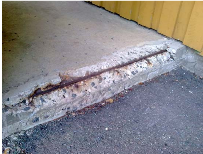
Fig.1.3. Typical reinforced concrete pavement slab damaged by wear
