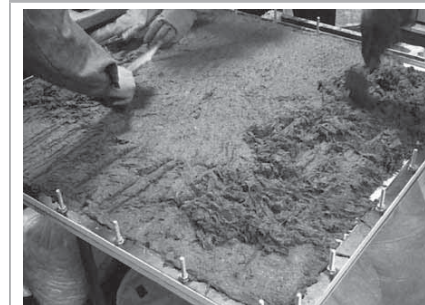
Figure 1. Short glass fiber concrete is evenly placed on the surface of rubber membrane (pneumatic mould).
