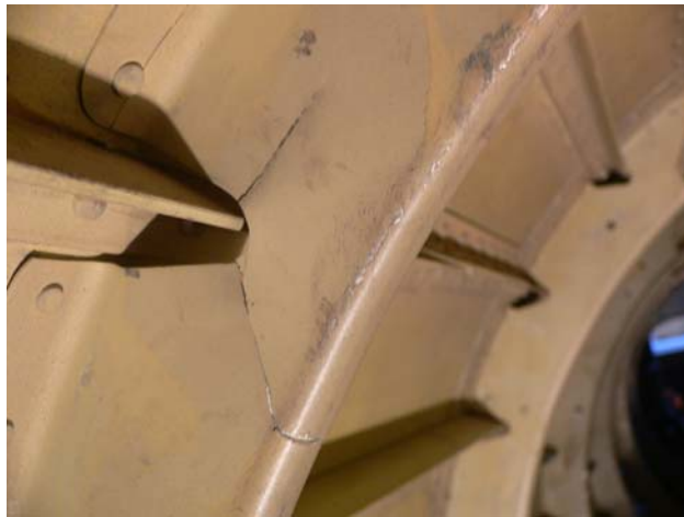
Fig. 6. The fatigue cracks in a frame as a result of dynamic overload induced by additional concentrated weight in middle part of the tail beam
