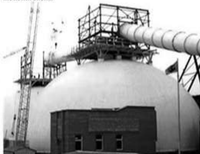
Fig.1. Ventspils, Kalija parks, whereas warehouses are made of fibro concrete, in shape formation there are used pneumatic formwork
