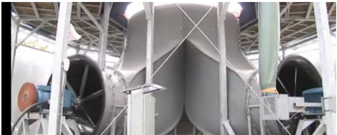
Fig. 3.21. Full-scale plant in Jelgava (Latvia).
