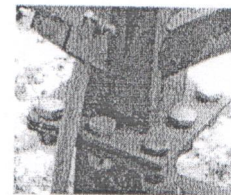
Fig. 3. Typical damage for steel structure
