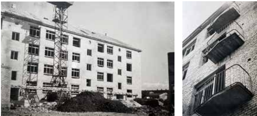
Figure 31. Construction of a residential building of the 1-430 series standard project in Liepāja, Brīvības Street (1956).
